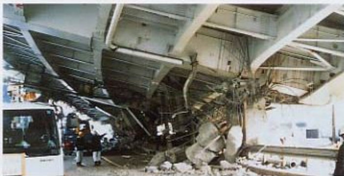
震災直後 Immediately after the earthquake
