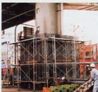
RC橋脚の2次災害防止のための応急補強 Emergency strengthening on a reinforced concrete pier for secondary disaster prevention
