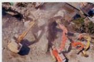
巨大なハサミで寸断される高速道路 Expressway structures being cut and removed using large scissors-like machines
