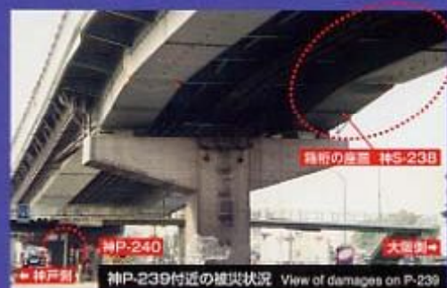
神P-239付近の被災状況 View of damages on P-239
