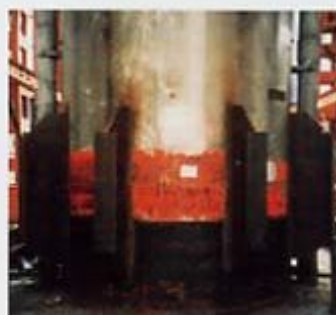
鋼製橋脚の2次災害防止のための応急補強 Emergency strengthening on a steel pier for secondary disaster prevention
